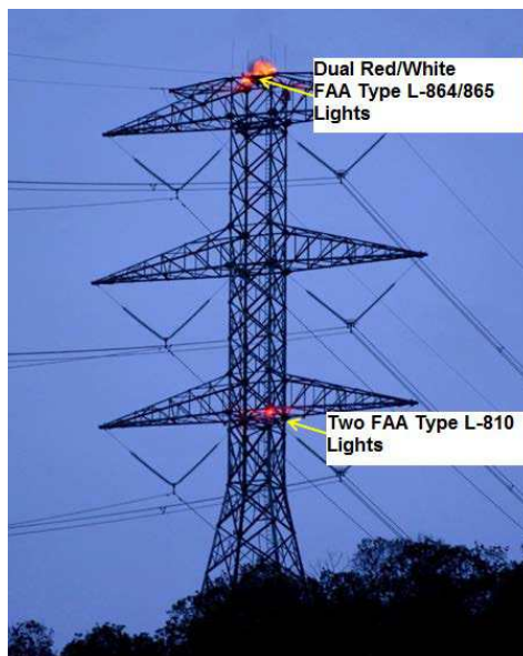
Figure 16. The FAA Type L-864/L-865 Obstruction Lights Controlled by the HARRIER ADLS [3]
