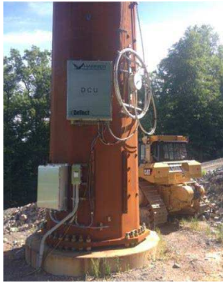
Figure 15. The DCU Installed on Transmission Tower [6]
