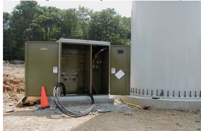
Figure 2.2.3.4-1 Typical Pad Mount Transformer (shown during construction before terminations landed)
