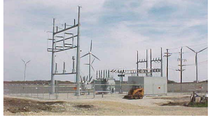
Figure 2.2.3.5-2 Typical Step-Up Substation
